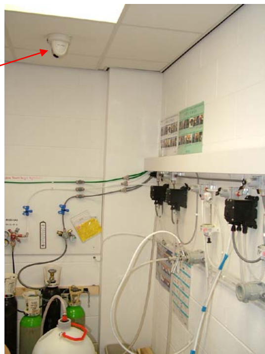
The Cellar Room with its ceiling mounted Elmo PTC450
