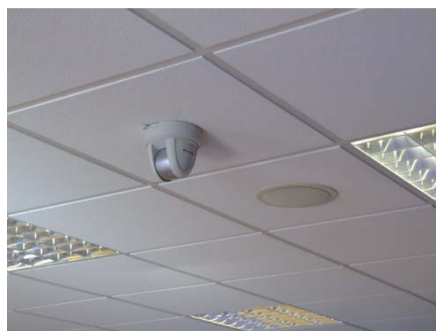
Photo of ceiling mounted speaker and Elmo PTC450 (Each camera records to central recorders in Server Rack and has a local button control pad for different views etc)
